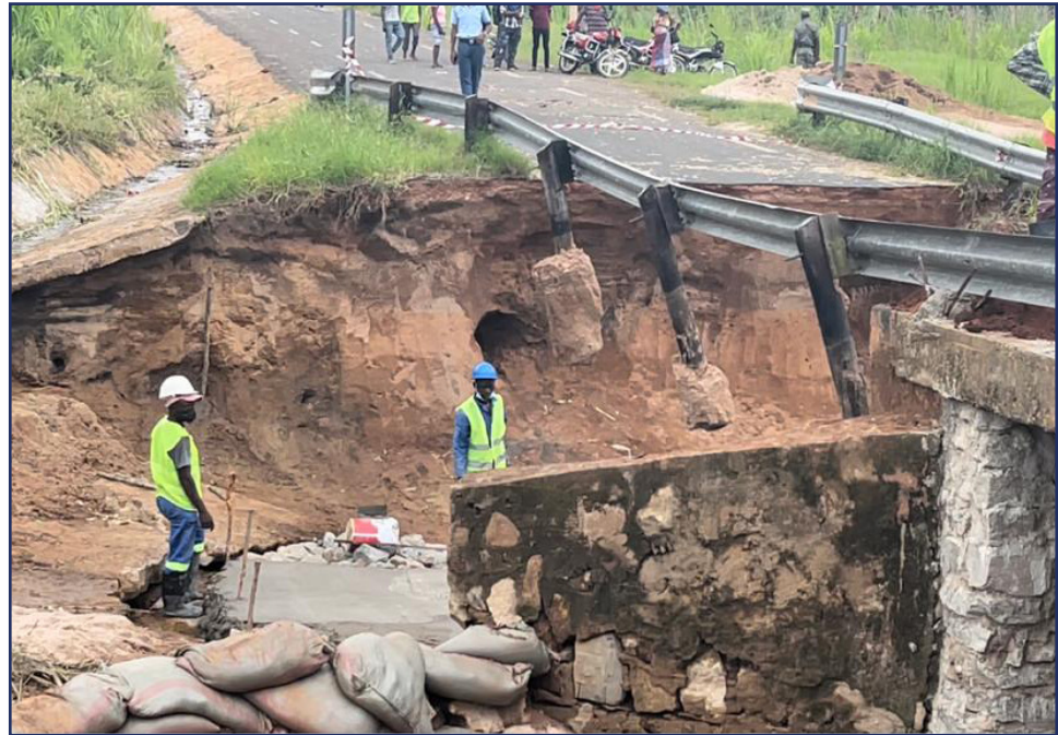
Extreme events have brought down roads and bridges in Zambézia and elsewhere in the country!
